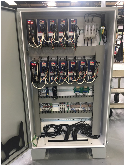
Multi-Spindle control enclosure
